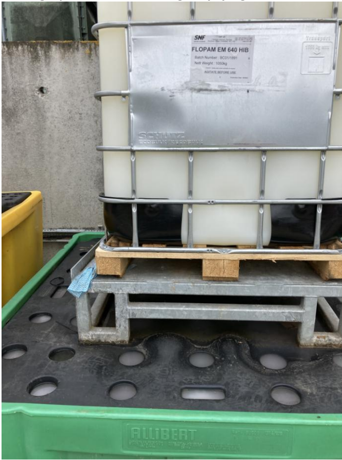
Photograph 1 - Bund needing emptying
